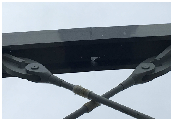
Figure 38: View of the hanger attachment close to an arch splice on the construction site
