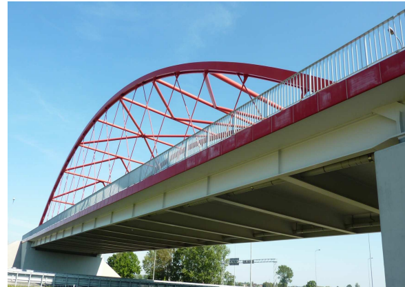
Figure 34: Bridge WD-57 in Rawicz (PL) over expressway S5 (Poznań – Wrocław) – 75m span [38]
