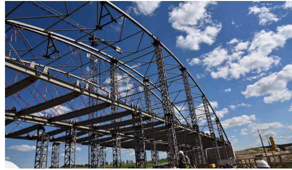
Figure 41: Erection of the arch segments by welding in its final position - MS-15 across the Łyna, - span 120 m
