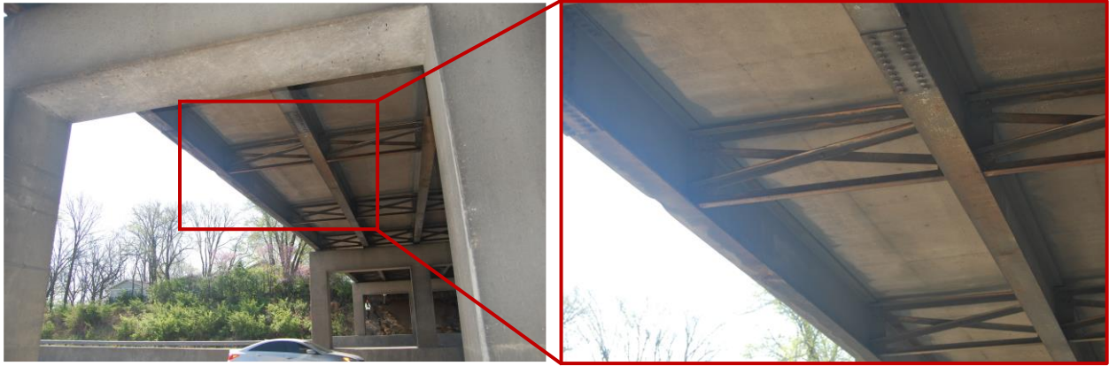
Figure 16. Underside view of the bridge from Figure 15 with coating deterioration in regions over the roadway.
