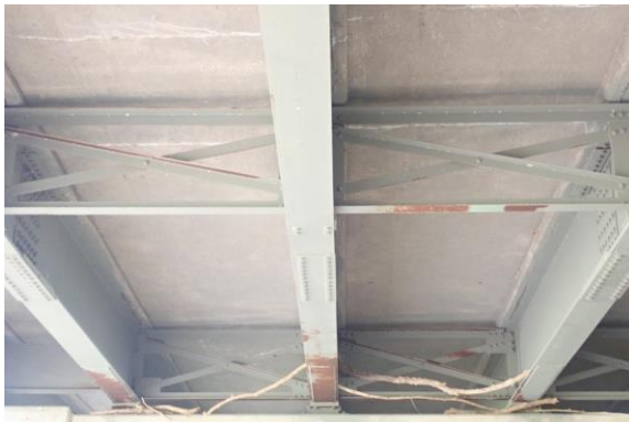
(c) edges and bottom surfaces of cross frames, undersides of bottom flanges
