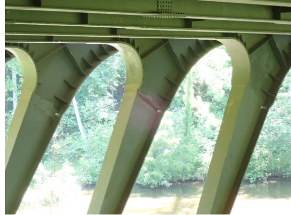
(b) location of corrosion
