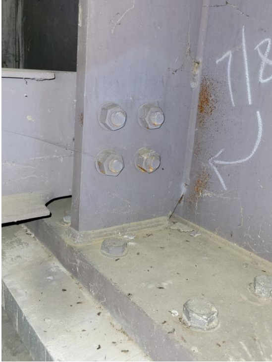
(a) insufficient coating and missed surfaces of a field coated bolted connection
