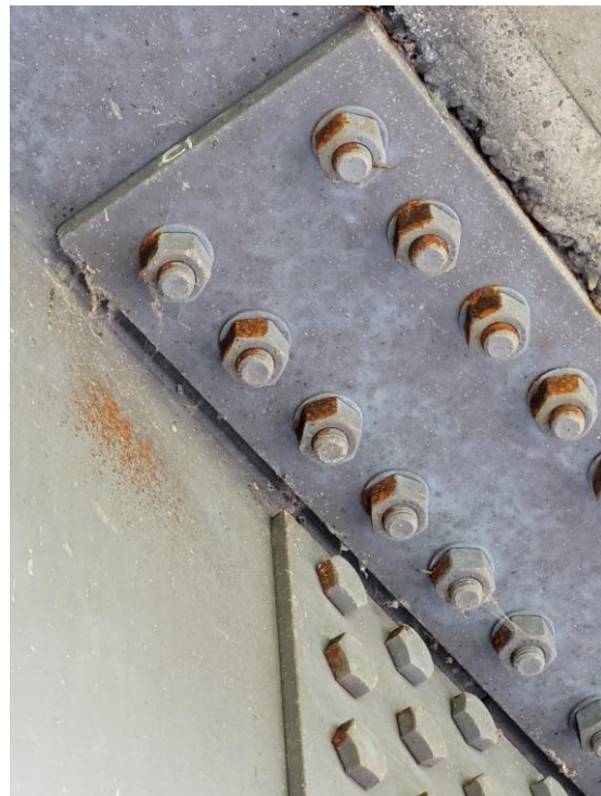
(b) surfaces of a bolted splice that were missed during field coating application
