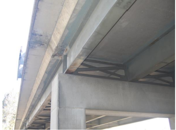
(b) deck overhang deterioration allowing unintended drainage onto the fascia girder resulting in coating failure and corrosion
