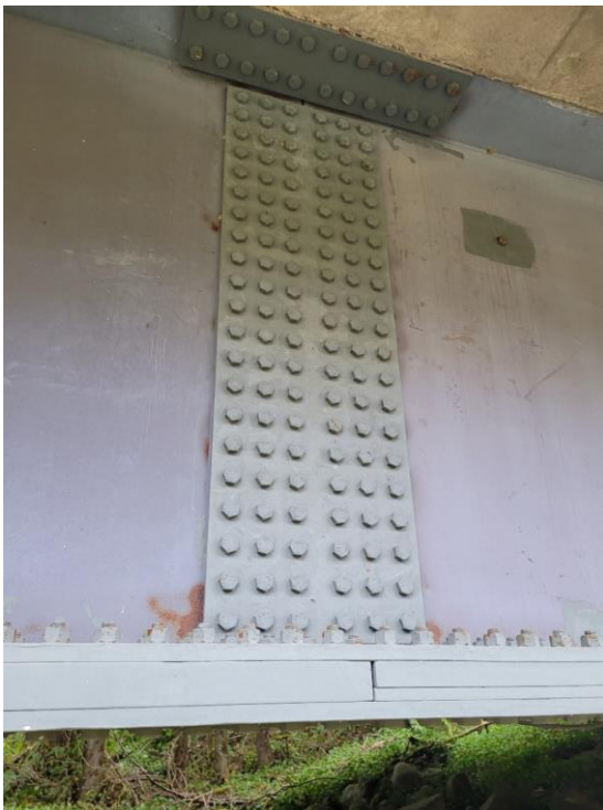
(a) bolted splice that was insufficiently coated over bolts and along plate edges
