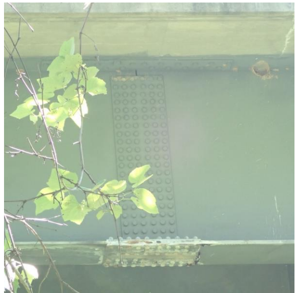
(d) bottom flange splice coating deterioration and steel corrosion caused by the same deck joint failure from (c)
