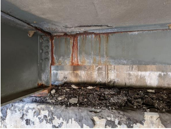
(a) efflorescence and corrosion of end diaphragm, connection plate, girder, and bearing plate
