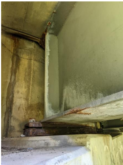
(c) efflorescence and corrosion of girder, bearing stiffener, and bearing plates
