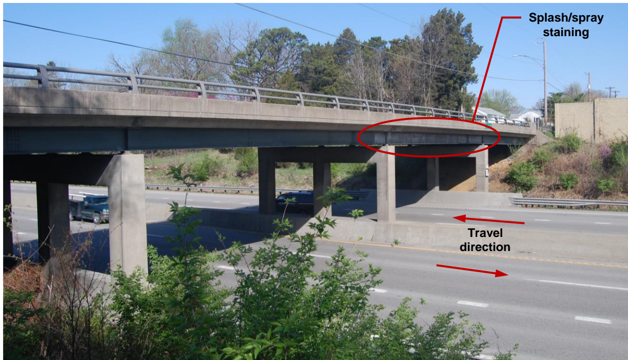
Figure 15. Roadway splash/spray zone.
